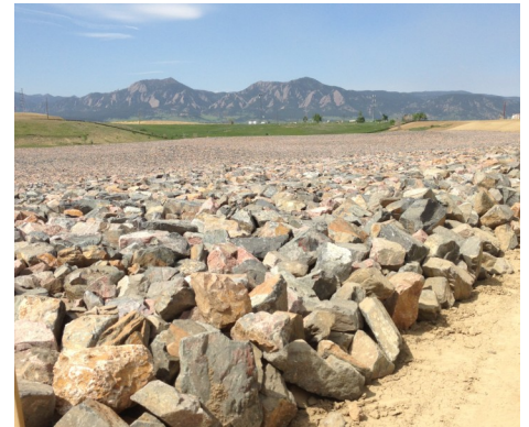
The rock cap completed as part of the Valmont Butte voluntary clean-up Program.
